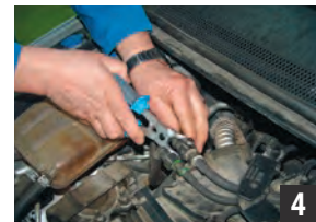
To couple fuel lines, clamps of plastic materials are used; with metal clamps, a spark might go off.
